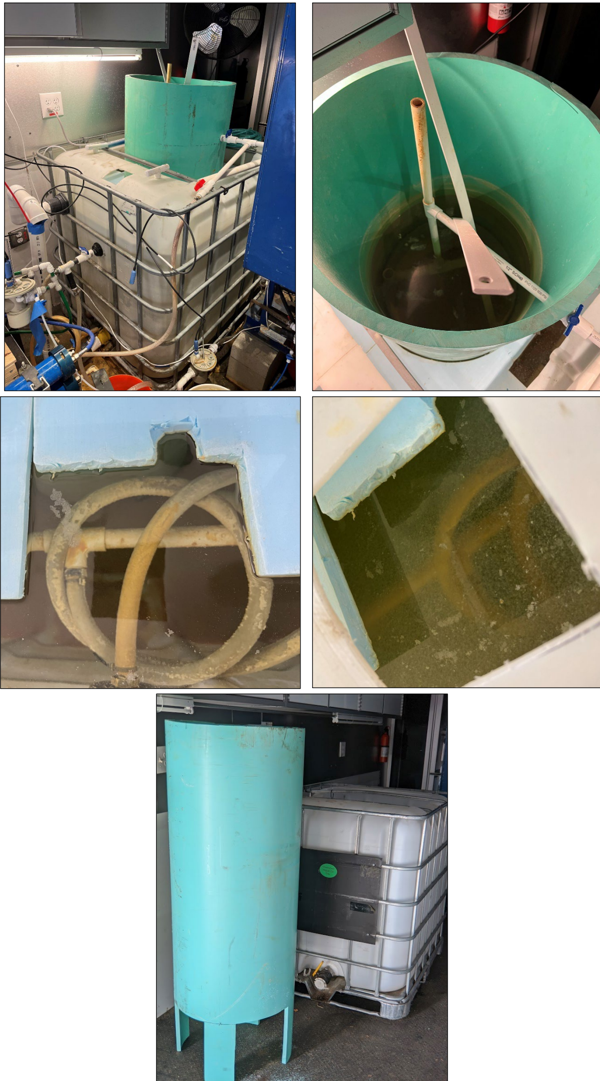
Figure 13.—Pictures of underflow clarifier.
