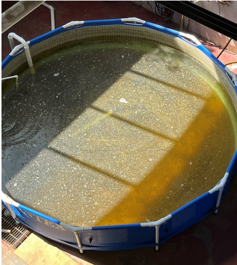
Figure 6.—Picture of blowdown capture pool during failure mode analysis (FMA) with significant algae growth.
