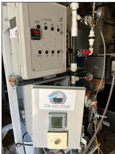
Power quality monitor and rheostat to control electrical load to heater
